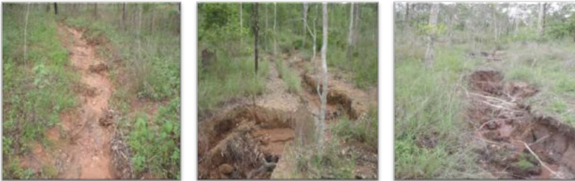
Figure 4 Examples of gullies emanating from road drains within the study area. 42% of road drains in the study area were found to have gullies like this associated within them
